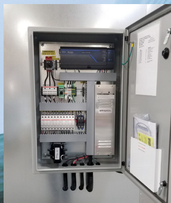
PLC Control System delivers highest degree of controlled precise operation and reliability.
